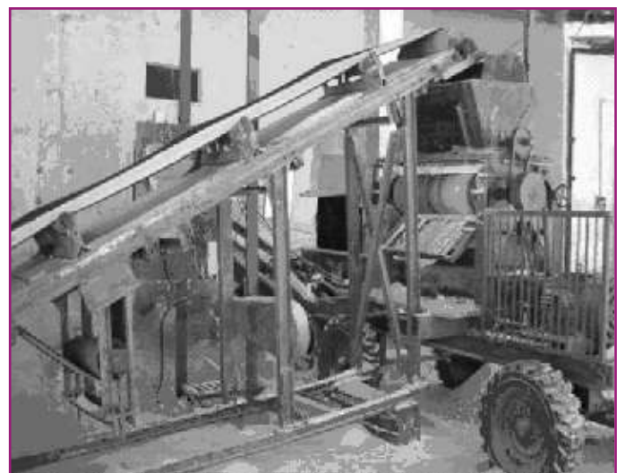
Iodized Salt Plant in Andhra Pradesh Identified for Repair
